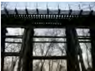
A RELIC FROM RAILROADING'S PAST: Though they pose a maintenance challenge, the Colebrookdale Railroad's bridges provide spectacular examples of early railroad engineering and, as contributing feature's to the line's unique character, should be considered assets.
