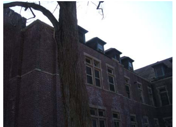
Limerick Hall Missing Coping
