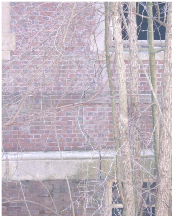
Vincennes Hall Wall Crack
