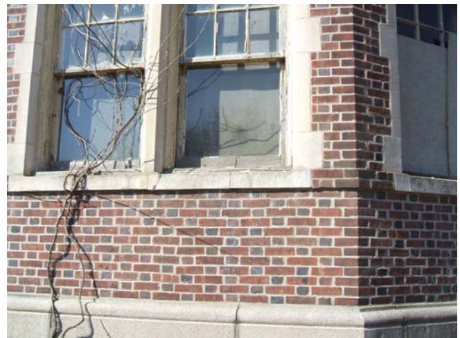
Industry Hall Vines and Cracked Limestone Sill
