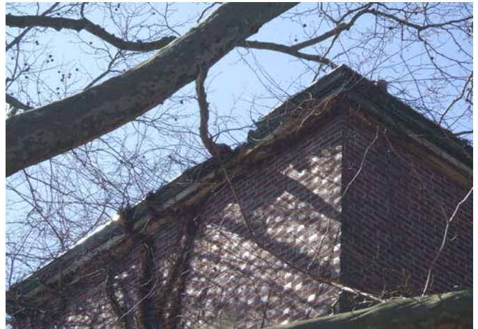
Tree Encroaching Upon Vincennes Hall
