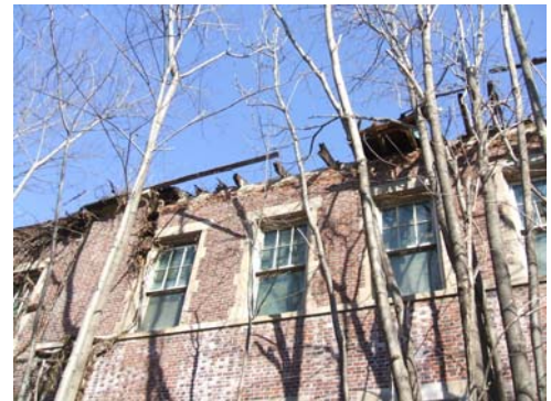
Hospital Cornice and Collapsed Roof
